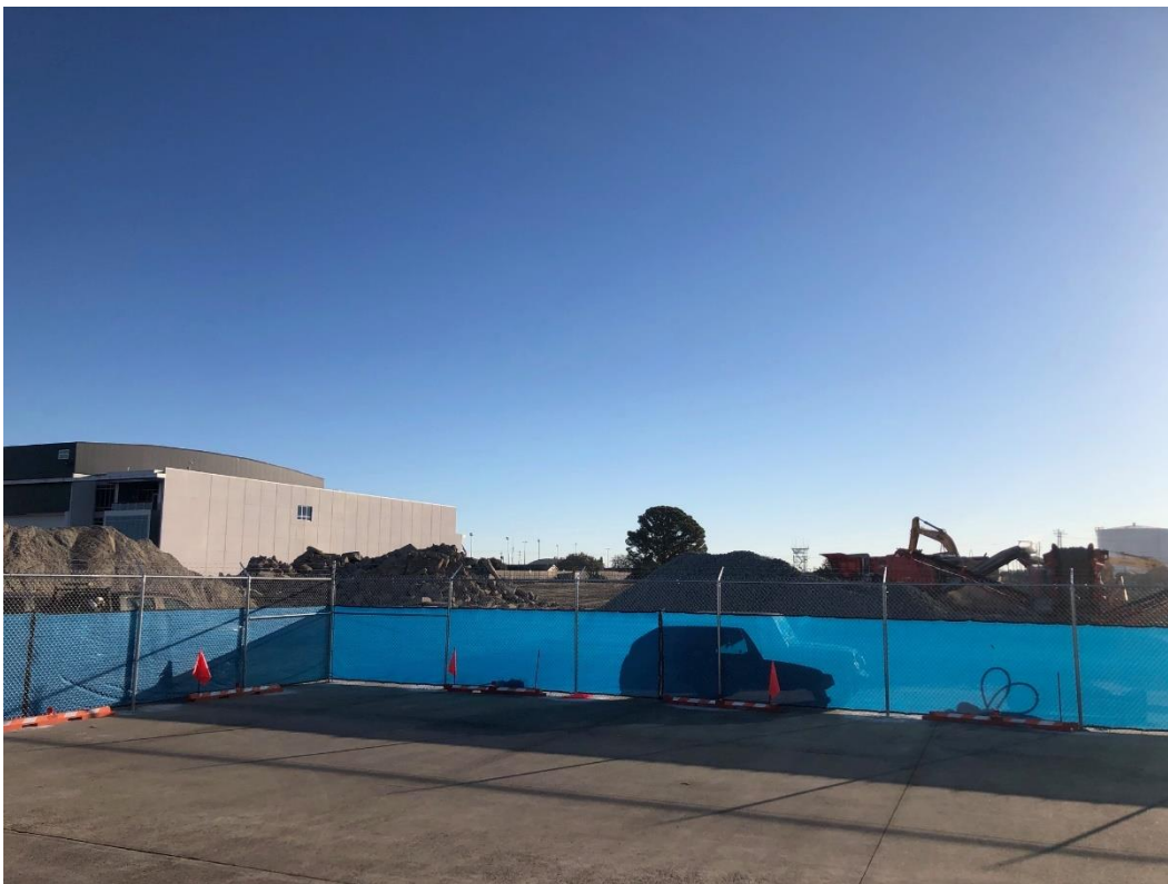
Figure 1: Demolition work is almost complete at the site of the old Signature FBO Building
